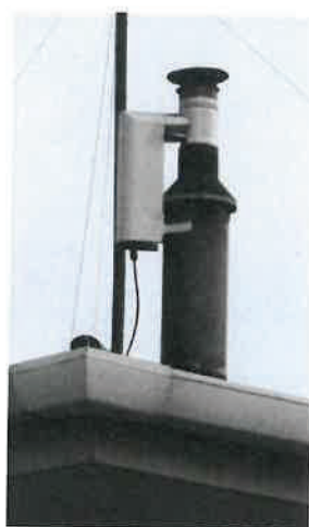
OekoTube circuit box on chimney
