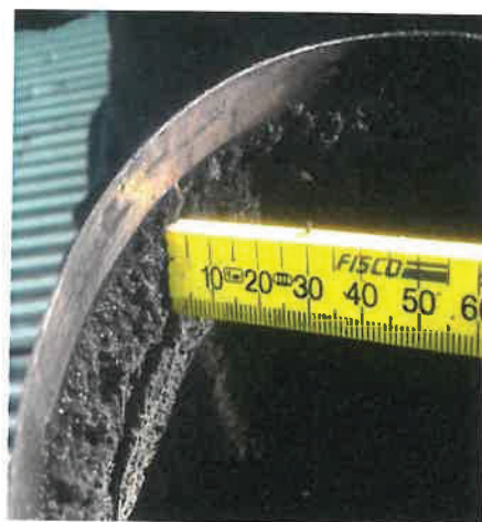
Coal dust 0.5mm thick on upper flue wall, 3 September
