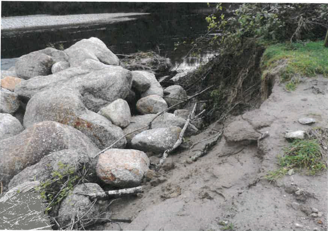
Photo 1: erosion scour behind spur – looking upstream.
