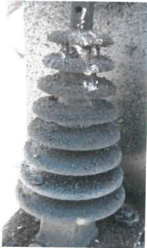
Insulator on coal fire, third monitoring round, 28 July. Note damage on top ring, discussed under 'Cleaning the firebox' on Page 8
