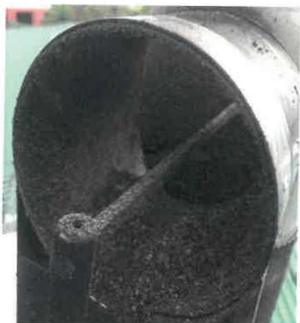
Black coal soot 1-4mm thick on upper flue wall, 0.1mm on electrode, 27 June
